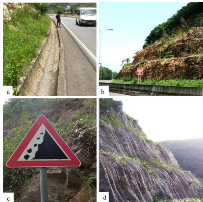
Figure 4. Rock fall Adaptation measures along the Peduase-Ayi Mensa road a) ditch and drain b) benches c) rock fall warning signs d) installed wire mesh Source: Field data (2017)
